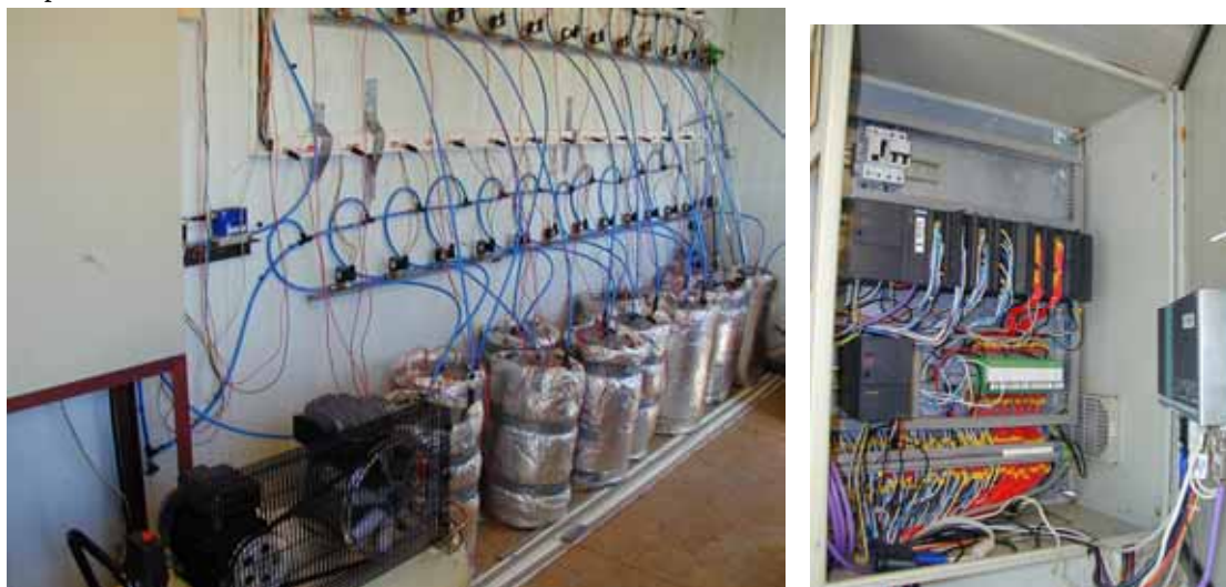
FIGURE 2 General view of the composting system (left) and control and monitoring system
